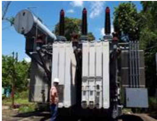
RETIRED TRANSFORMER UNIT 1 – 22MVA
