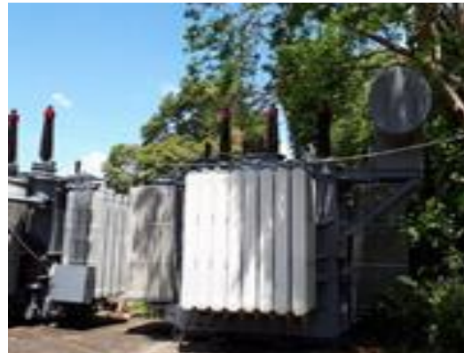
RETIRED TRANSFORMER UNIT 2 – 22MVA
