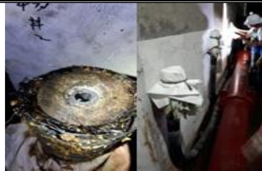
RETIRED 230KV OIL FILLED CABLES
