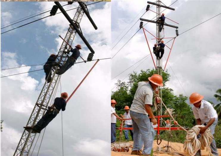
Top photo shows the Angat hydroelectric power plant. Below, technical crew undertakes maintenance and upgrading operations for the transmission lines.
